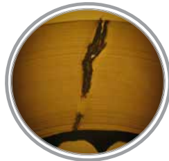
Image: partial discharge failure
